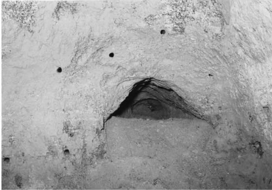
Photograph 12A. Results of Burn Cut Number 12. Bottom of Drilled Cut is Visible in the Picture.
