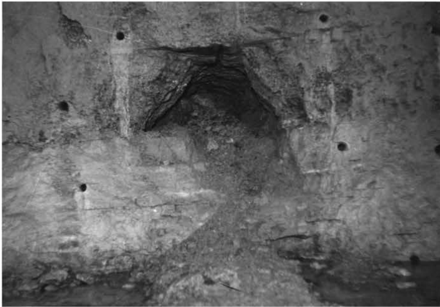
Photograph 5. Results of Burn Cut Number 5 Bottom of Cut is 9\frac{1}{2} Feet From Original Face.
