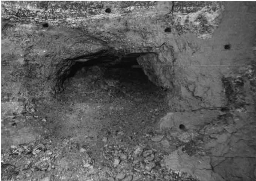
Photograph 9. Results of Burn Cut Number 9. The Bottom of the Cut is 9'9" From the Original Face of the Drift.
